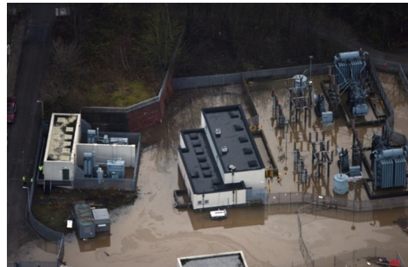
Flooded power station at Lancaster in December 2015
