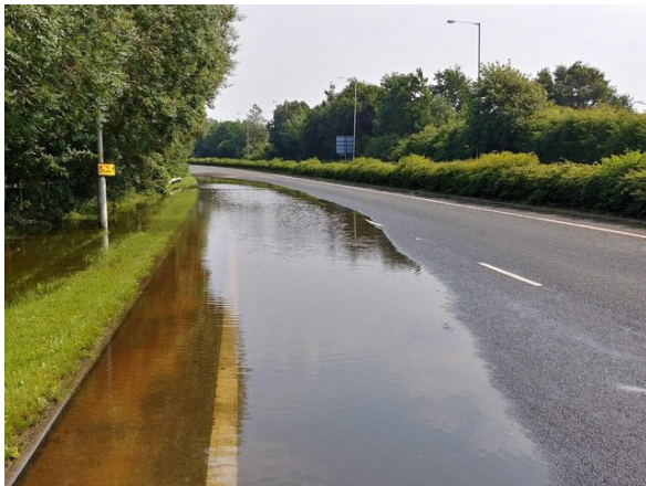
Highway flooding on the A584 in Freckleton 11 August 2020
